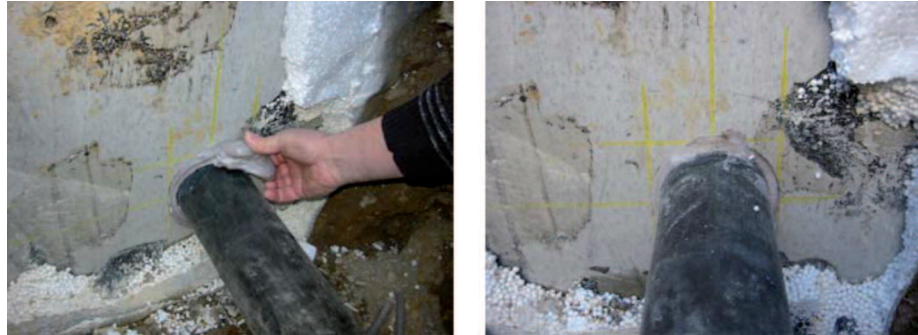
Fig. 5 Removing the Tangit M 3000 expansion resin and the PE cord (left), finished seal (right).
