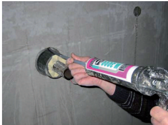
Fig. 6 Filling the cavity on the basement side with Tangit M 3000 expansion resin
