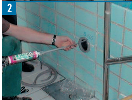
2 Injection of the Tangit M 3000 Expansion Resin from the inside of the pool wall.
