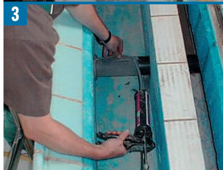
3 Injection of the Tangit M 3000 Expansion Resin from the outside of the pool wall.
