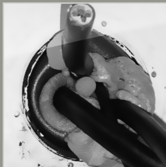
...insert the pipe and seal it on both sides with M 3000 – finished!
