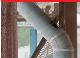
Pipes and Ducts
