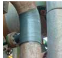
Pipe Work and Valves
