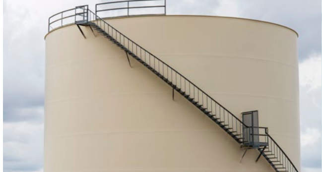
With concrete protection
