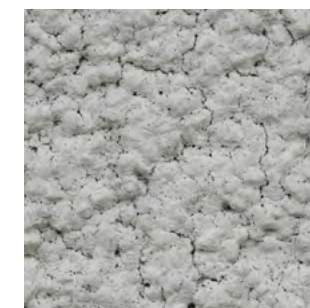
Render with micro-cracks
