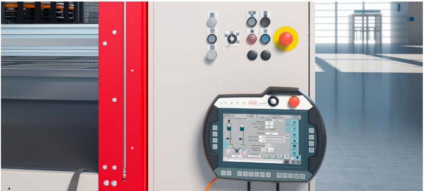
MP 2 mobile panel and above it the operating mode control panel, e.g. key switch for operating mode preselection with selection for the operating modes of Setup / Stand-by / Manual / Automatic, warning lights and EMERGENCY STOP, part of the tried-and-tested SONDERHOFF SAFETY concept.
