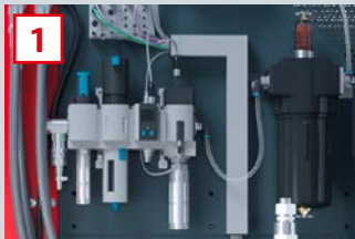
Compressed air connection, dryer and maintenance unit
